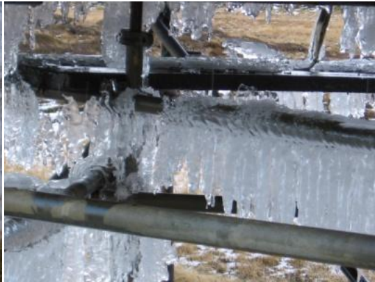
Frozen water underneath water tanks
